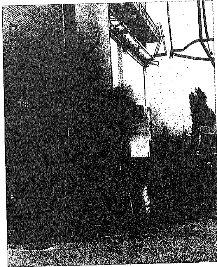
Photo 3 - Aspect of the prefabricated substation and indicators in the test circuit after test from IAC A
